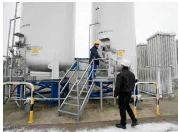
At Ketzin, just outside Berlin, Germany, CO2SINK is a joint project between 18 companies and institutes from nine countries developing the basis for CCS storage by injecting CO2 into a saline aquifer. (Photo courtesy European Commission )
